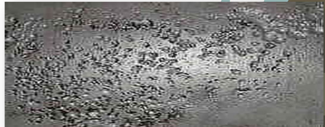
Corrosion and wall thinning in a pipeline Source: NDT.net
